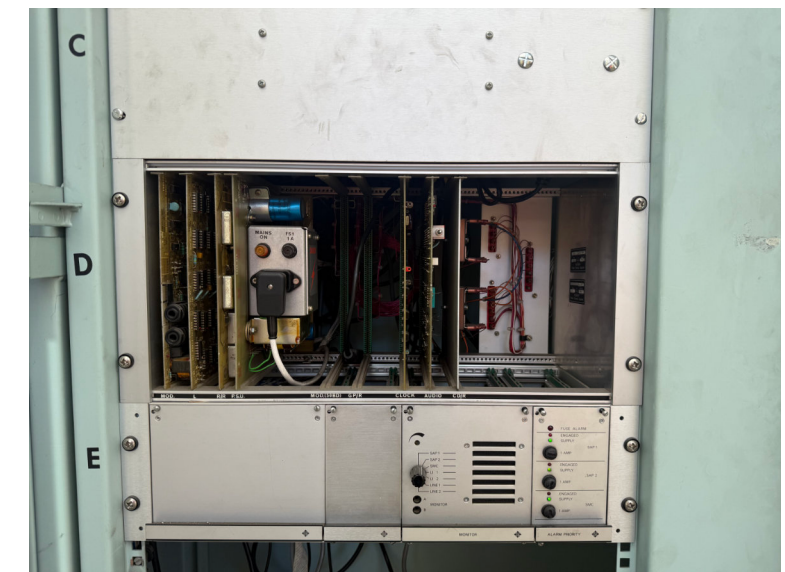
Fig 5.18.5.1-1: Existing PA Central Equipment
