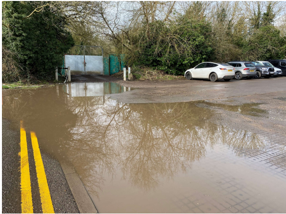
Current condition of the carpark during times of heavy rain.
